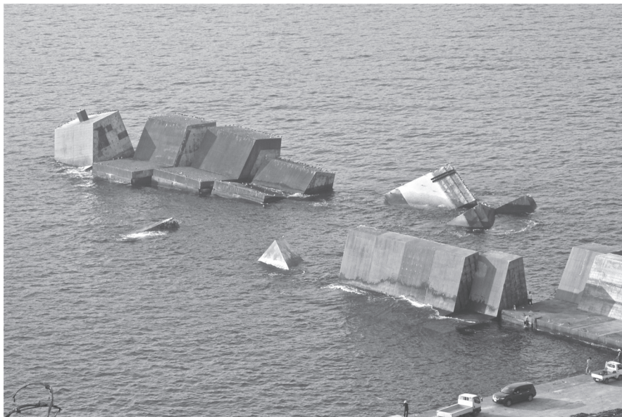
Fig. 5; A seawall in Tohoku, destroyed by the tsunami of March 11, 2011.
